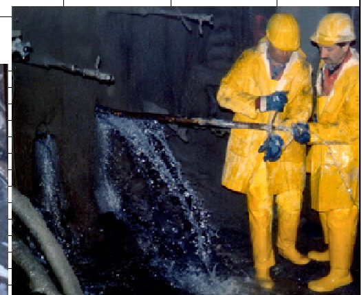
Expert advisor, water ingress in tunnel, Füssen, Germany
